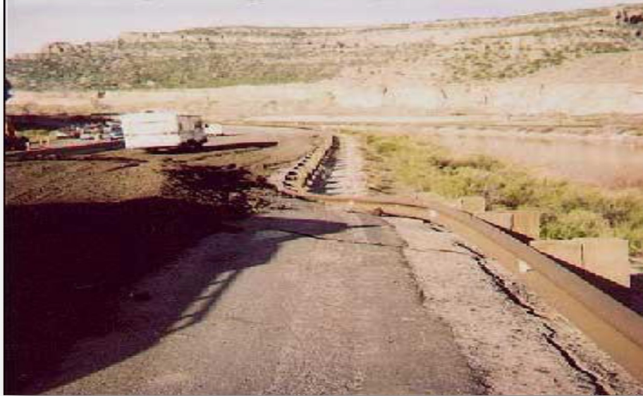
FIGURE 11 PHOTO OF DeBEQUE CANYON SLIDE AREA- INTERSTATE 70
