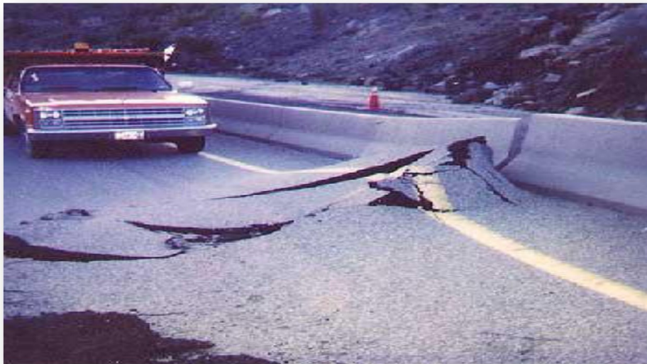
FIGURE 12 PHOTO OF DeBEQUE CANYON SLIDE AREA- INTERSTATE 70
