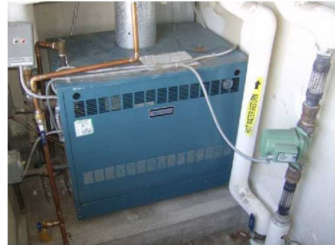
Existing Heating Water Boiler
