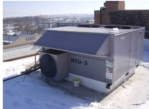
Existing Auditorium Rooftop Unit
