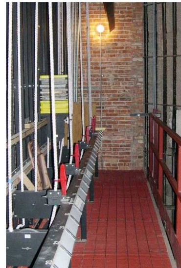
Stage Left Fly Gallery w/ Locking Rail and Counterweight Arbor
