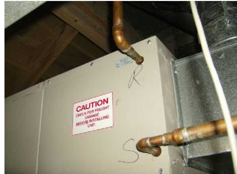
Typical Fan Coil Unit
