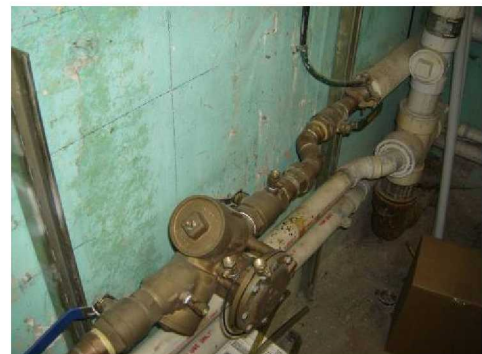
Existing Domestic Water Service
