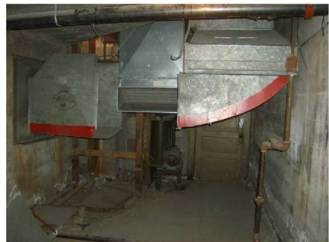
Original Air Distribution Ductwork in Basement
