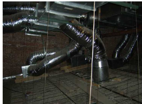
Typical Air Distribution above Auditorium
