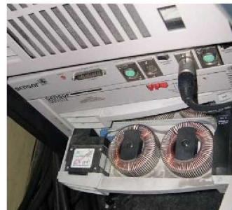
Dirt in Dimmer Modules
