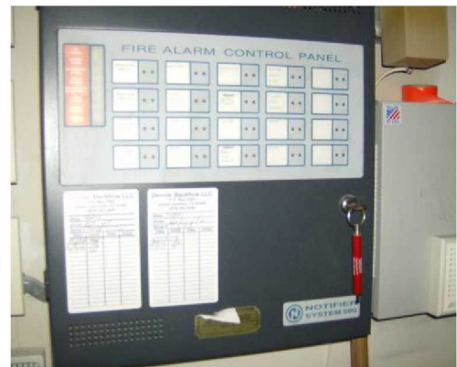
Existing Notifier System 500 Fire Alarm Control Panel
