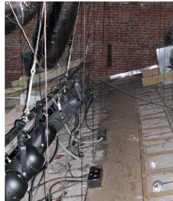
Existing Auditorium Ceiling Cove Stage Lighting Position
