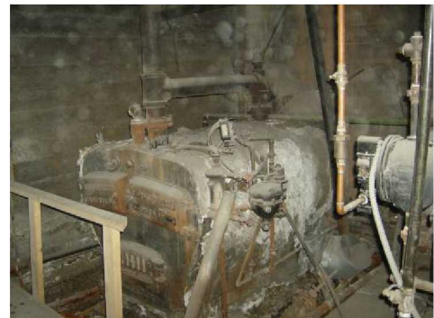
Original Steam Boiler
