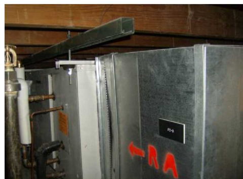
Typical Fan Coil Unit
