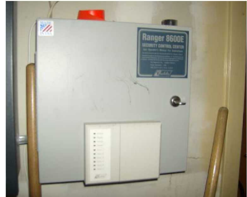
Existing Ranger 8600E Security Control Panel
