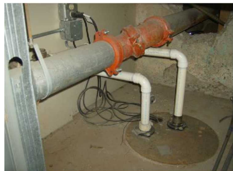
Existing Sump Pump
