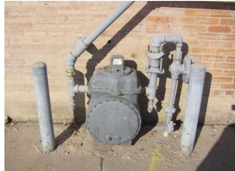
Existing Natural Gas Service and Meter
