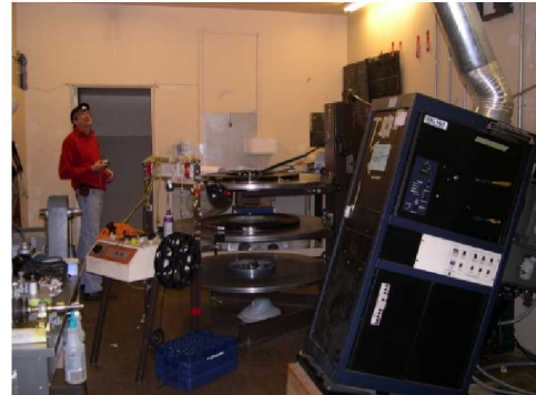
Humidifier underneath platter system
