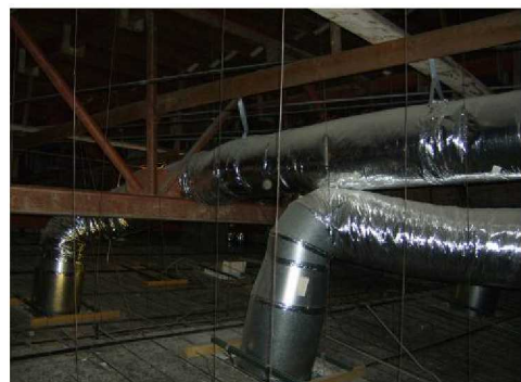
Typical Air Distribution above Auditorium
