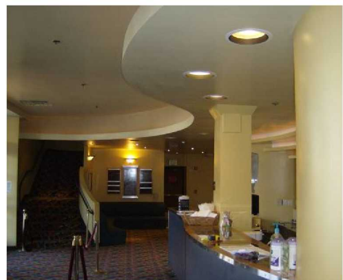
Existing Lobby Lighting
