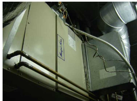
Typical Fan Coil Unit
