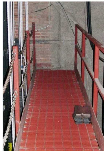
Loading Bridge w/ Few Counterweights
