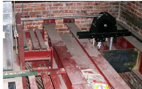
Unprotected Ladder Opening at Edge of Grid Iron
