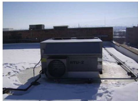
Existing Auditorium Rooftop Unit
