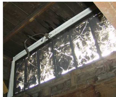
Unsecured Smoke Vent
