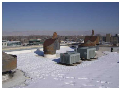
Air-Cooled Condensing Units associated with Fan Coil Units
