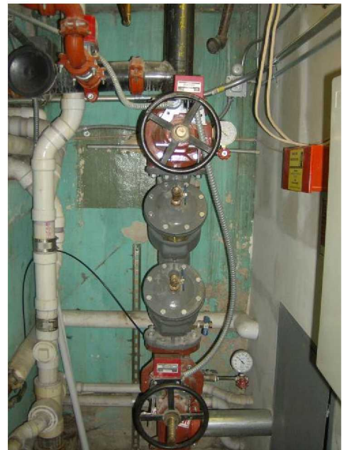
Existing Fire Protection Service
