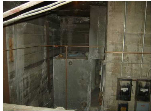
Original Water-Cooled Condenser
