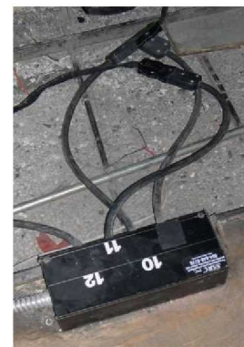
Auditorium Ceiling Outlet Box
