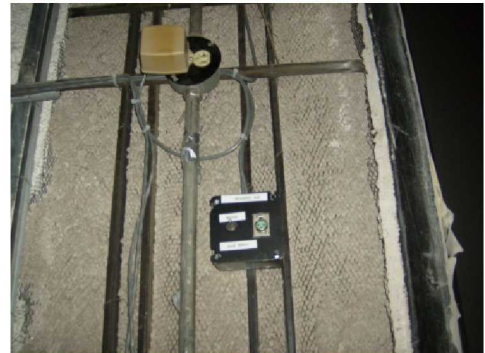
Mic cable wrapped around electrical conduit
