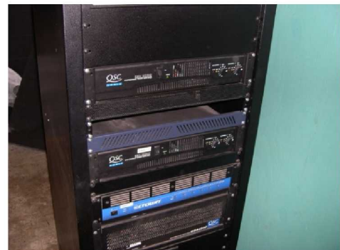
Amplifiers inside equipment rack
