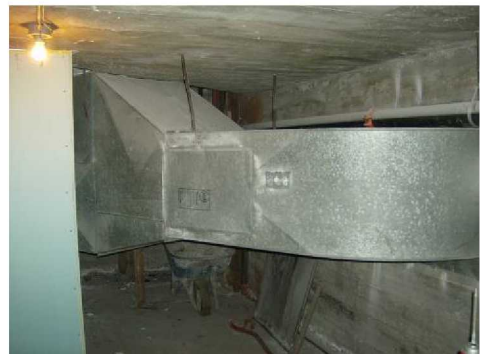
Original Air Distribution Ductwork in Basement
