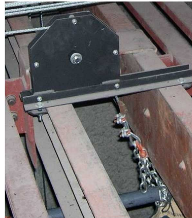
Misaligned Trim Chain Batten Connection
