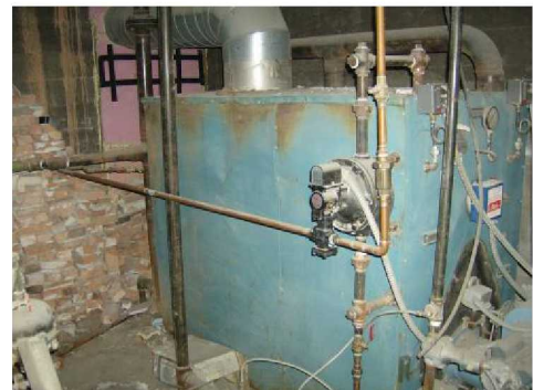
"Newer" Original Steam Boiler
