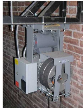
Acoustic Drapery Winch Motor
