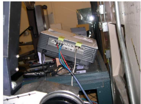
Component wiring to projector strained
