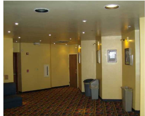
Existing Lobby Lighting
