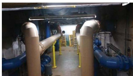
Photo 1: GI WTP Filter Pinina Gallery
