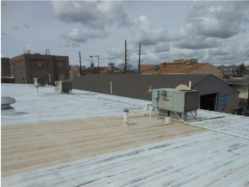
Photo #1: RTU-1, 2 and 3 from right to left.
