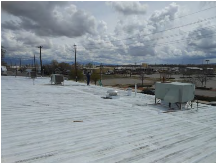
Photo #2. RTU-4, 5 and 6 from right to left.
