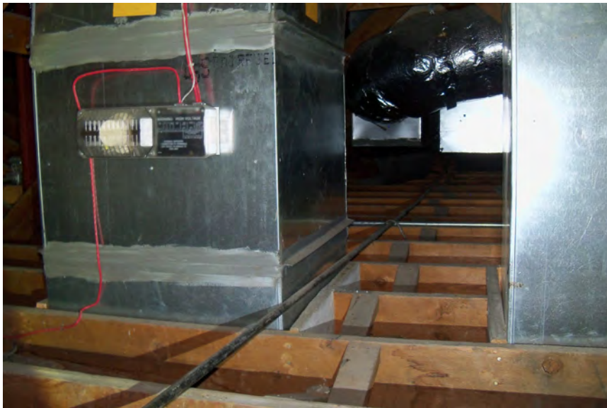
Typical attic space showing new HVAC ducting.
