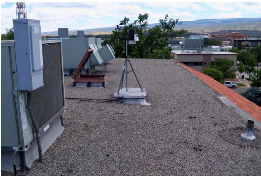
View to south from roof showing weather station, HVAC units, and flat and sloping portions of roof.
