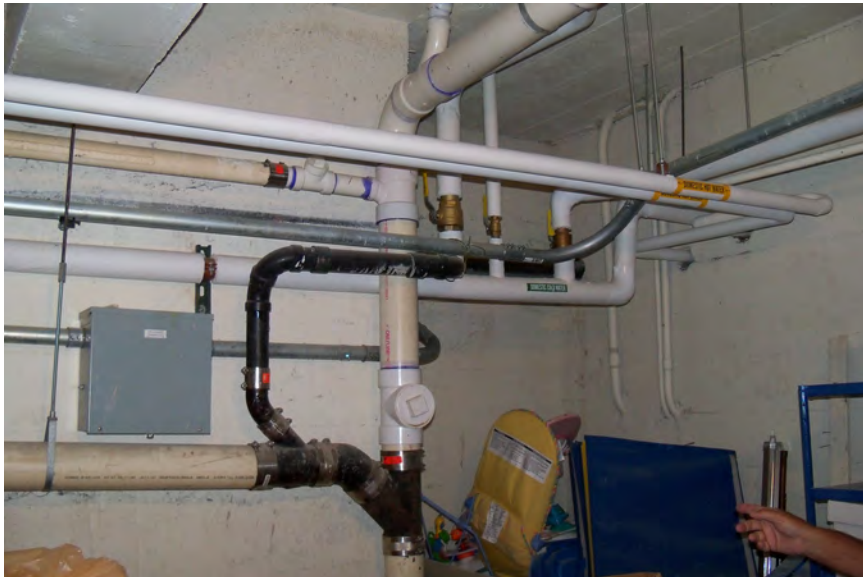
View of basement utilities
