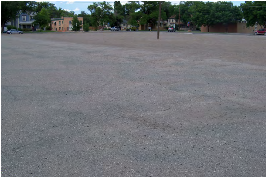
Parking area; paved in foreground and gravel in background. View to northeast.
