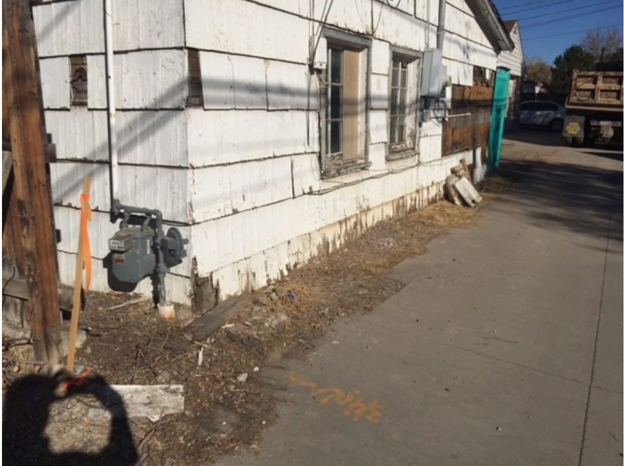
Existing building encroaching into the alley right-of-way Alley right-of-way is 20' wide with 16' of concrete Building does not encroach into the improved portion of the alley
