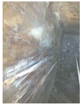
WET WELL NO. 1
