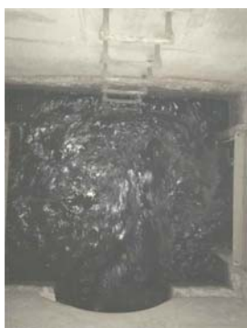
GRIT SPLITTER BOX NO. 2
