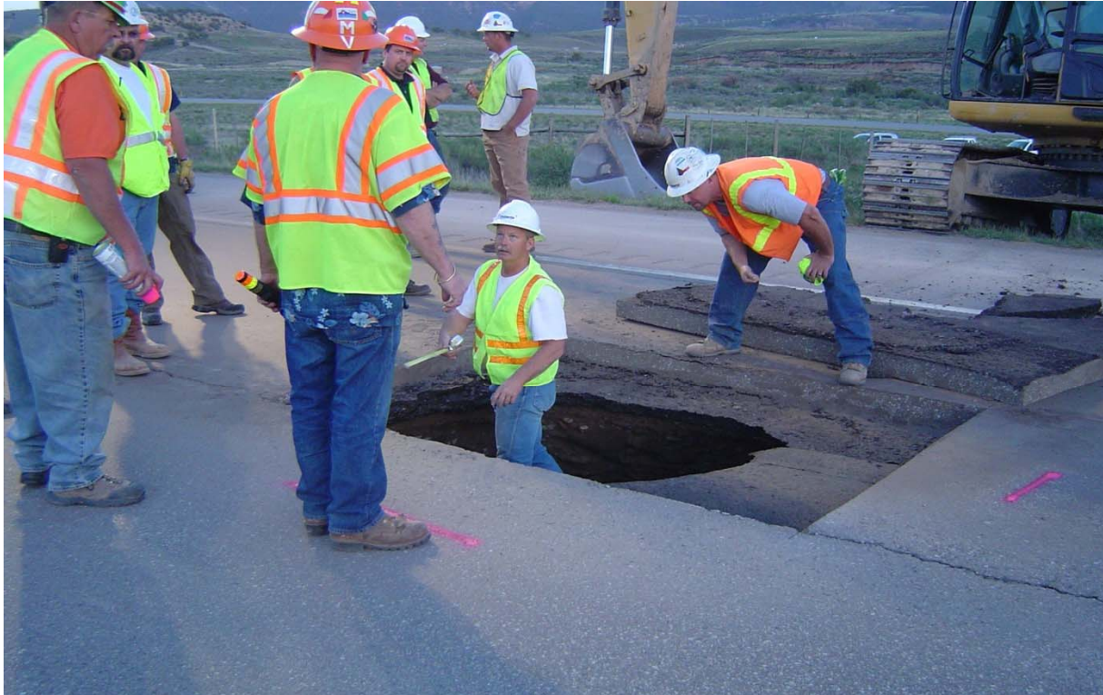
I-70 Eastbound lanes- Void resulting from incorrect construction of 20 inch High Pressure Gas bore
