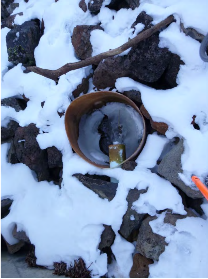
Photo 7: Collection and monitoring pipe from right side of outlet headwall.
