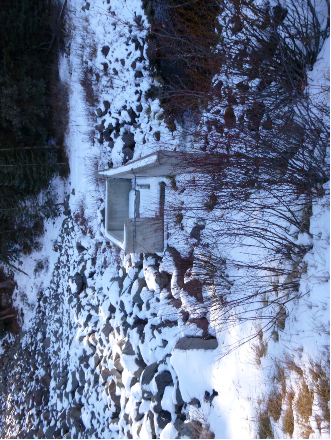
Photo 6: Abandoned outlet hydraulics control building foundation behind headwall.
