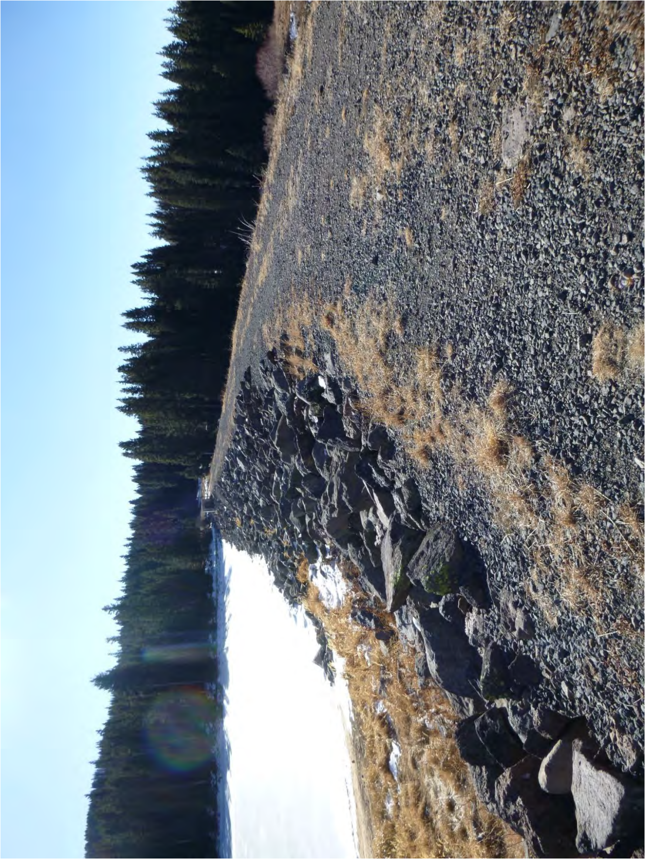
Photo 2: Upstream slope; Outlet hydraulics control building at center of dam on upstream edge of dam crest.
