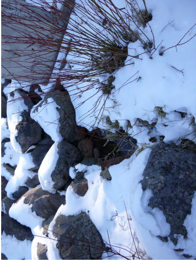
Photo 11: Seepage behind right side of outlet headwall.
