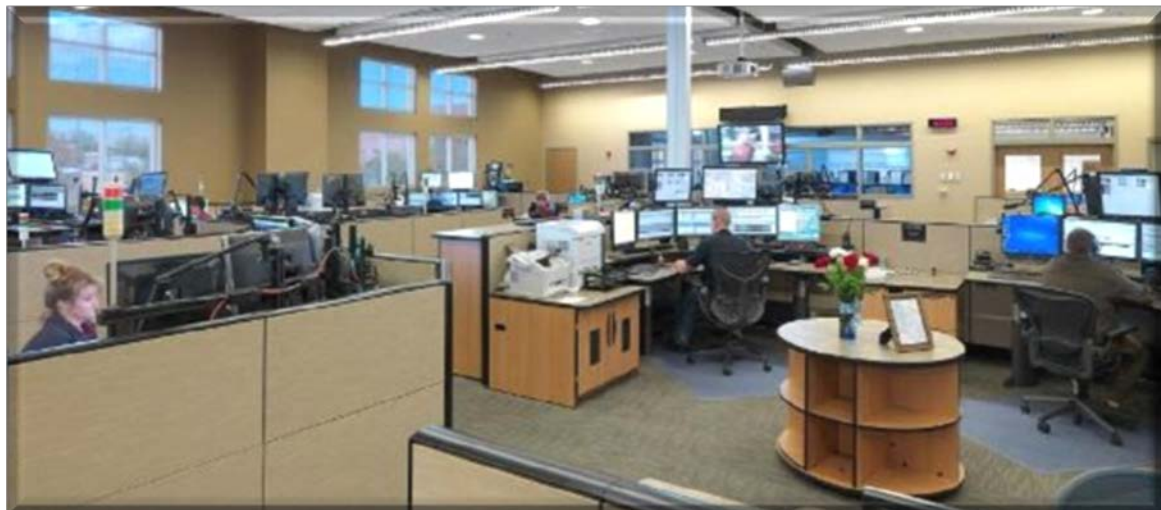
Grand Junction 9-1-1 Communications Center
