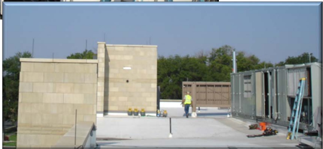
Air Conditioning Units Maintained by Facilities
