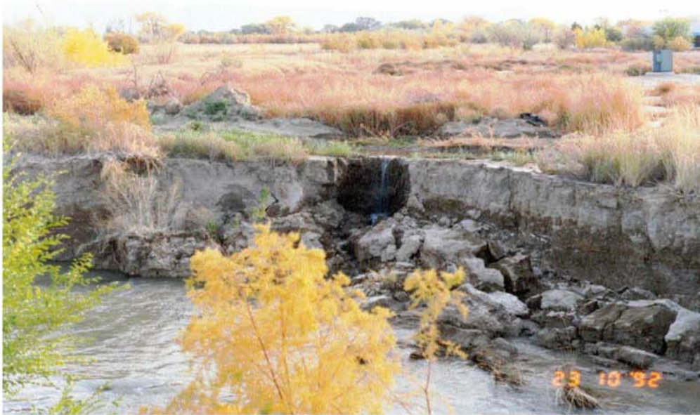
Figure 11. Bank Erosion in Leach Creek just North of F ¼ Road (North of Mesa Mall)
