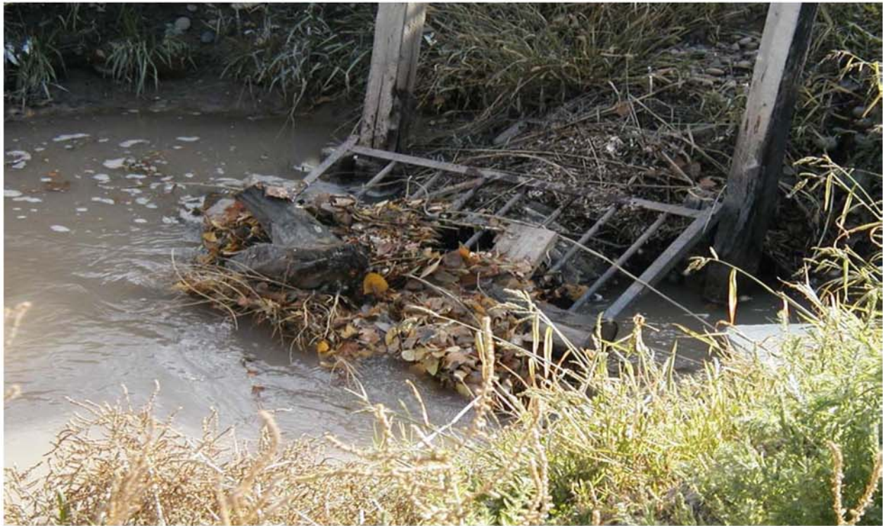
Figure 3. Example of Common Maintenance Needs
