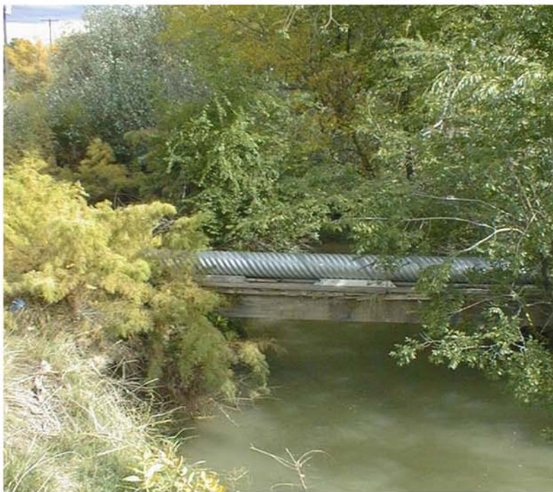
Figure 6. Utility Crossing and Overgrown Channel
