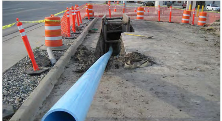
Fusible PVC was used for directional boring and pipe bursting the old ductile and cast water lines.
