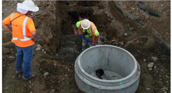
Installing a new sanitary sewer manhole. Many of the previous manholes were made of brick.
