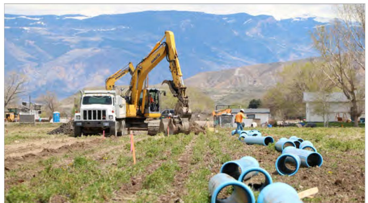
New 12-inch water main that will connect the new 400,000 gallon elevated tank to the town. This tank and line greatly improved fire flows and the dependability of their water system.
