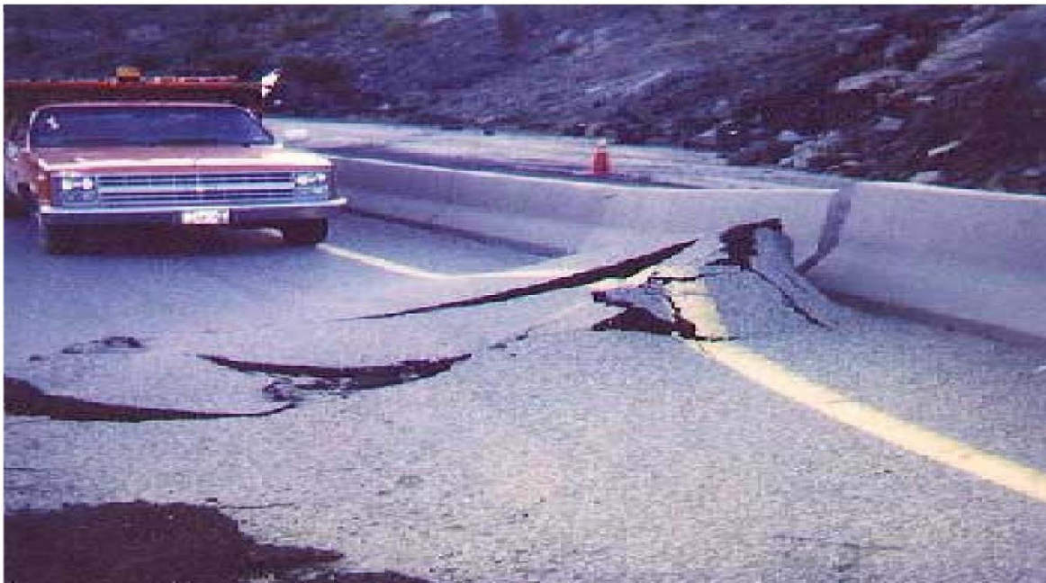
Figure 12: Photo of DeBeque Canyon Slide Area – Interstate 70
