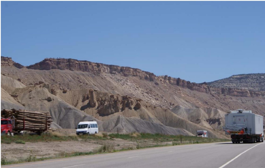
Figure 13: Rockfall West of Palisade Along Interstate 70
