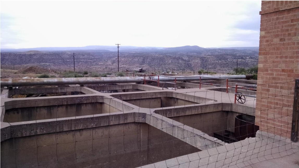
Filtration Basins and View to South
