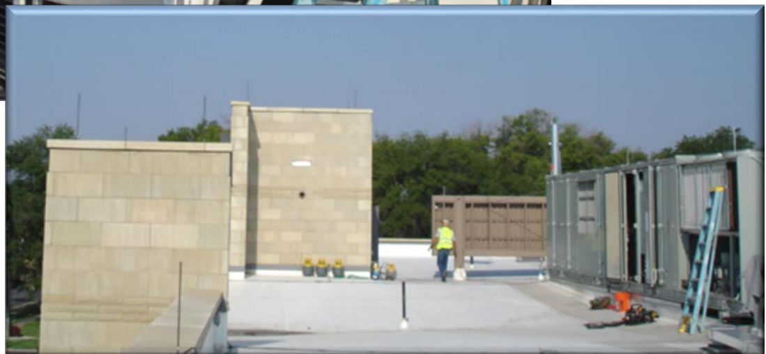
City Building AC Units
