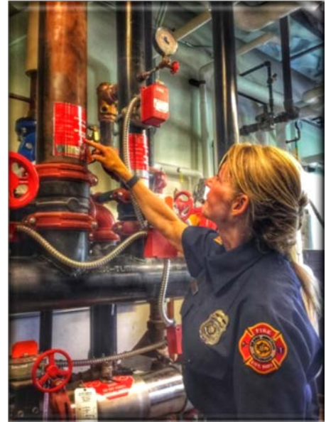
Fire Suppression Equipment Inspection
