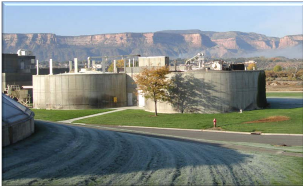
Persigo Wastewater Treatment Plant
