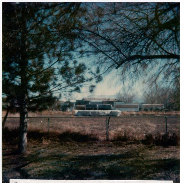
Construction yard with stacks of lumber beginning 125 feet east of applicant's property as represented by fence.
