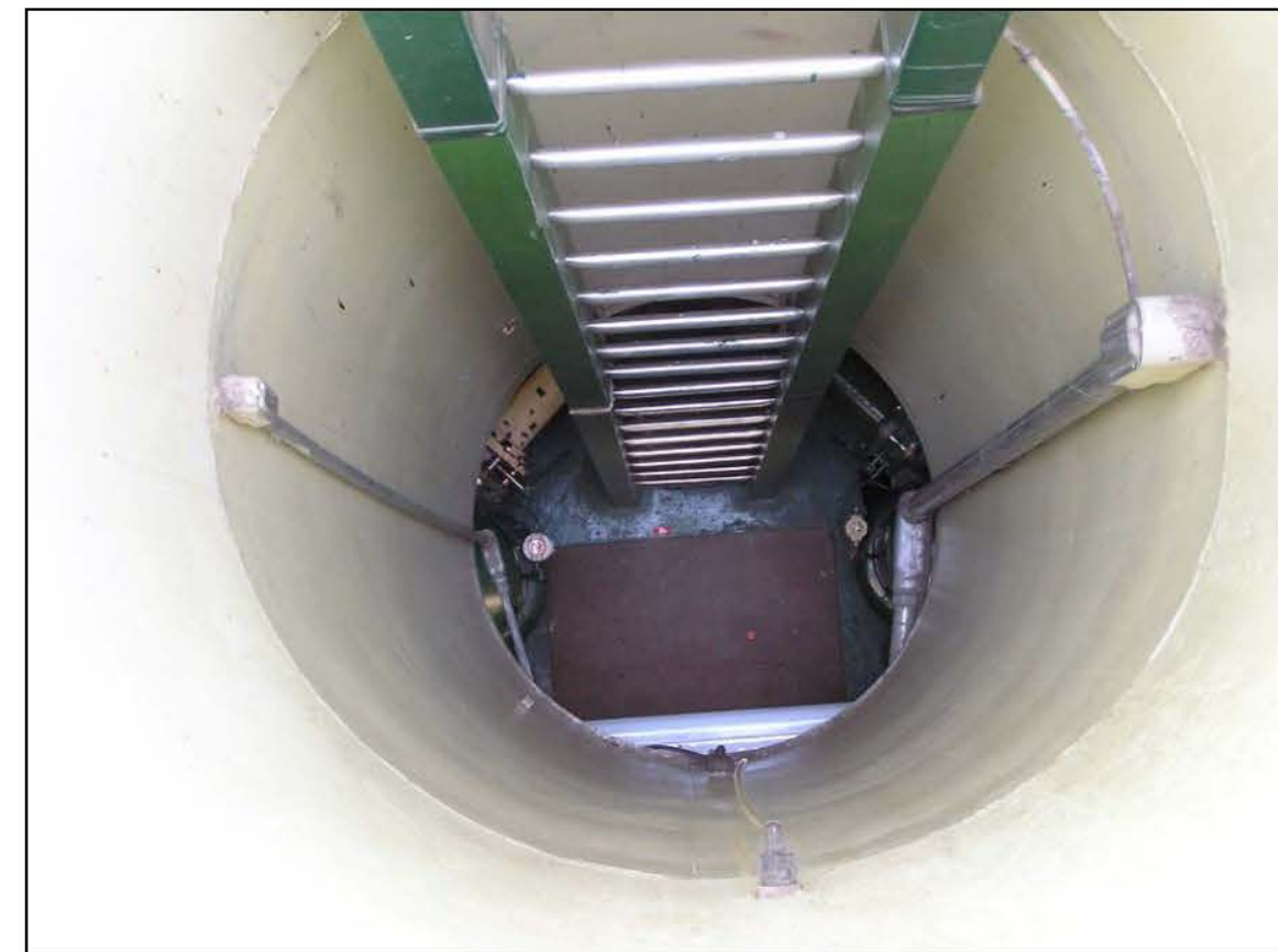
PHOTO B PEPSI LIFT STATION PUMP ACCESS TO BE REMOVED 3' BELOW GRADE & BACKFILLED AFTER CITY SALVAGE BY CONTRACTOR.
