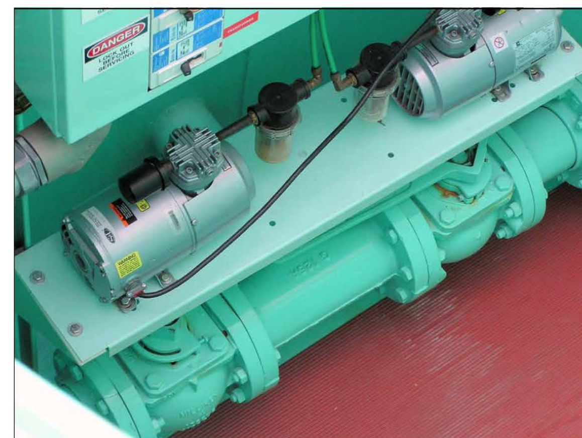
PHOTO D EXISTING ROSEVALE LIFT STATION PUMPS AND DISCHARGE PIPING
