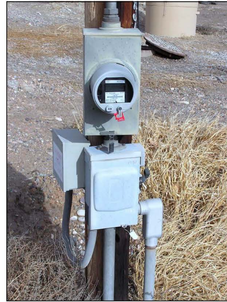
PHOTO A PEPSI LIFT STATION ELECTRIC SERVICE TO BE DISCONNECTED BY CITY AND XCEL ENERGY
