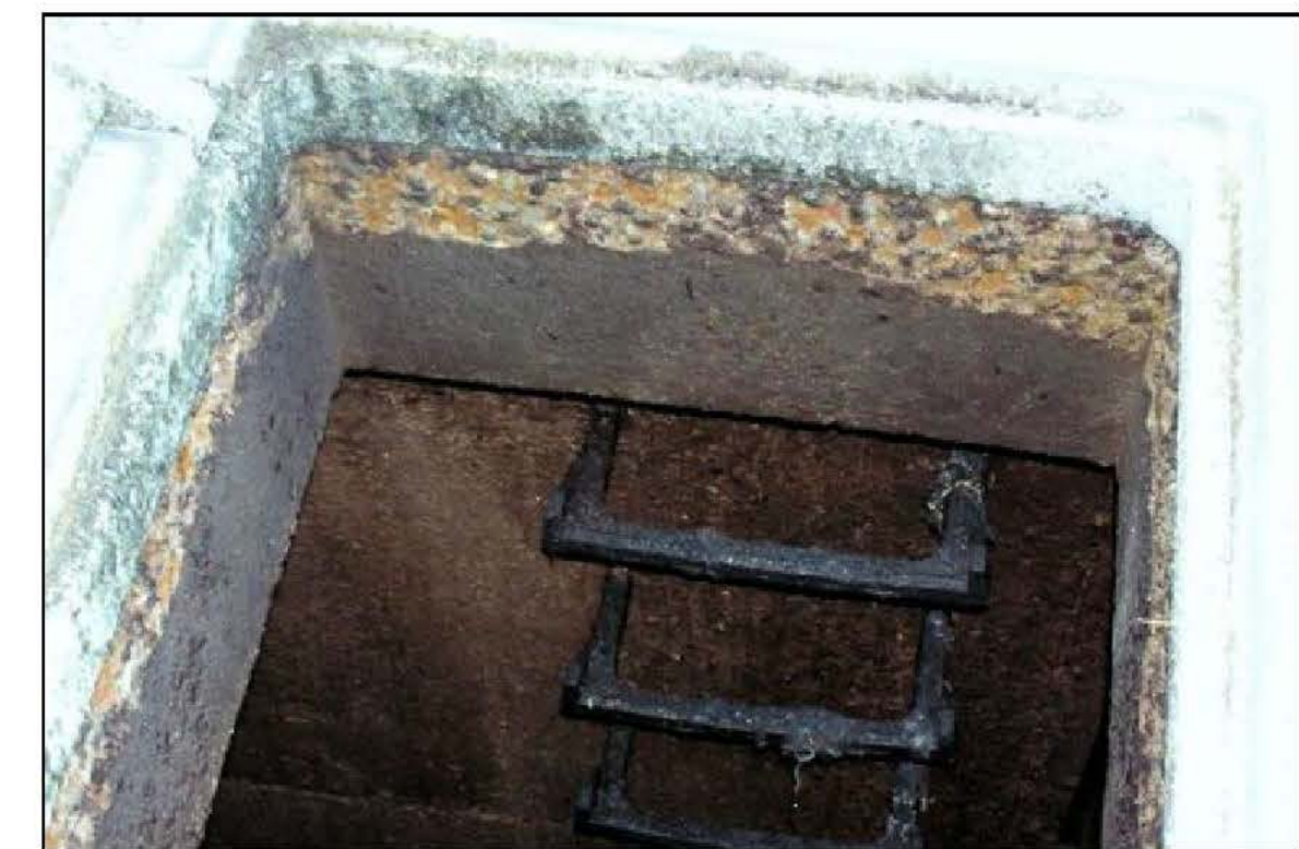
19 LOOKING WEST INSIDE WET WELL NO 2 AT WEST WALL AND ACCESS RUNGS
