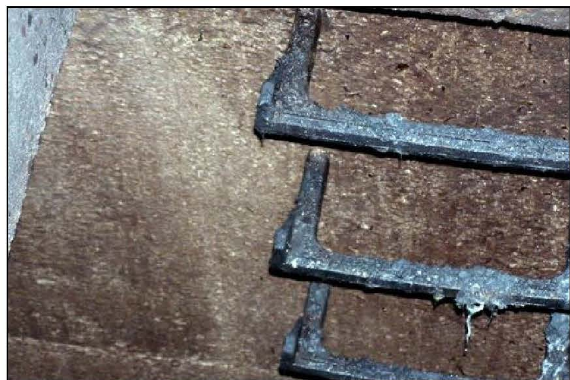
20 LOOKING SOUTH WEST INSIDE WET WELL NO 2 AT WEST WALL AND ACCESS RUNGS
