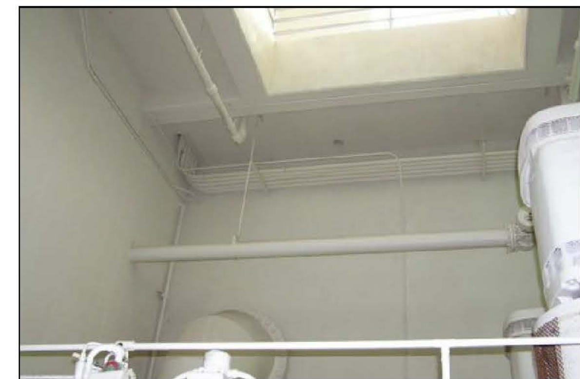
24 LOOKING UP AND EAST ACROSS PUMP ROOM AT 6" DUCTILE IRON PIPE FROM PRIMARY SLUDGE PUMP STATION AND 2" DRAIN PIPE
