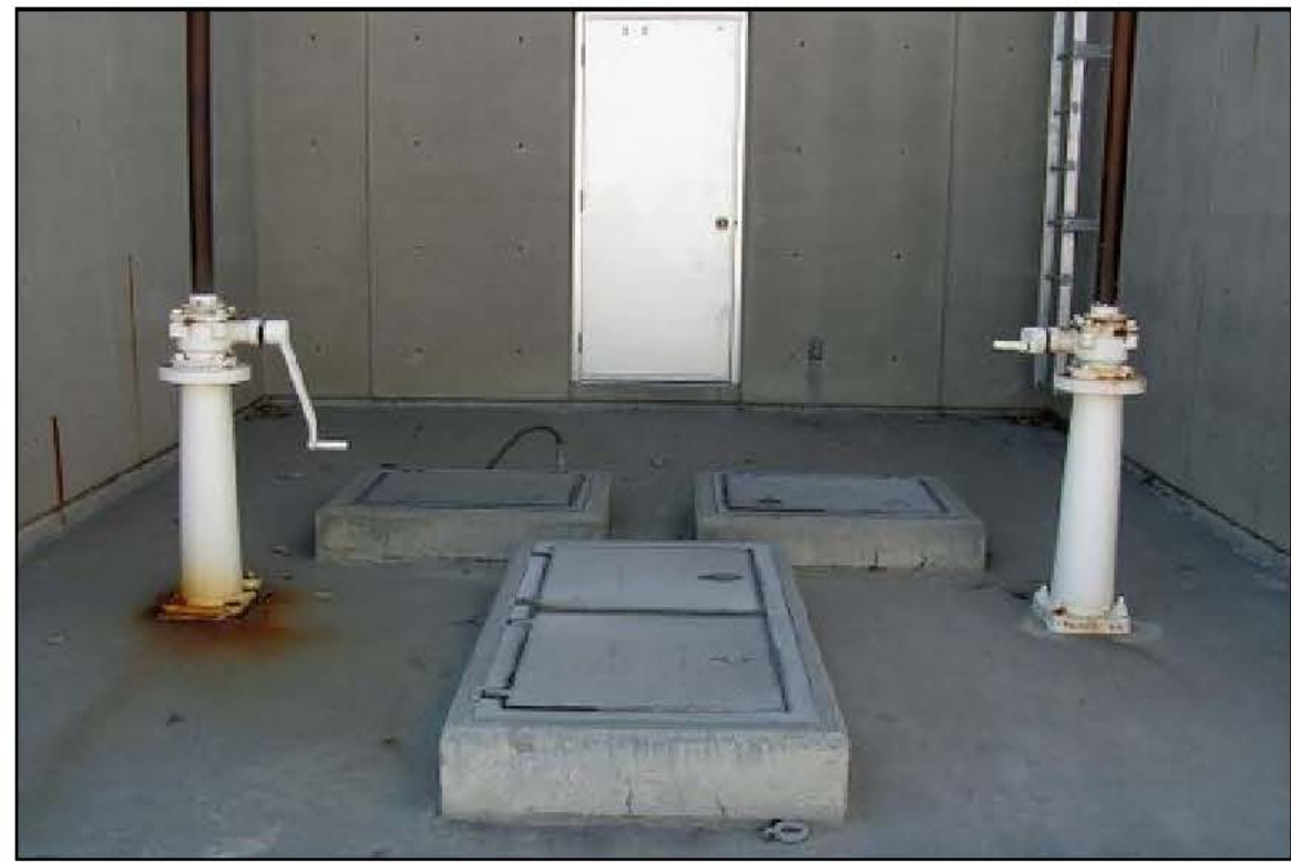
05 LOOKING SOUTH AT INFLUENT & WET WELLS ACCESS AND SLUICE VALVE CONTROLLERS
