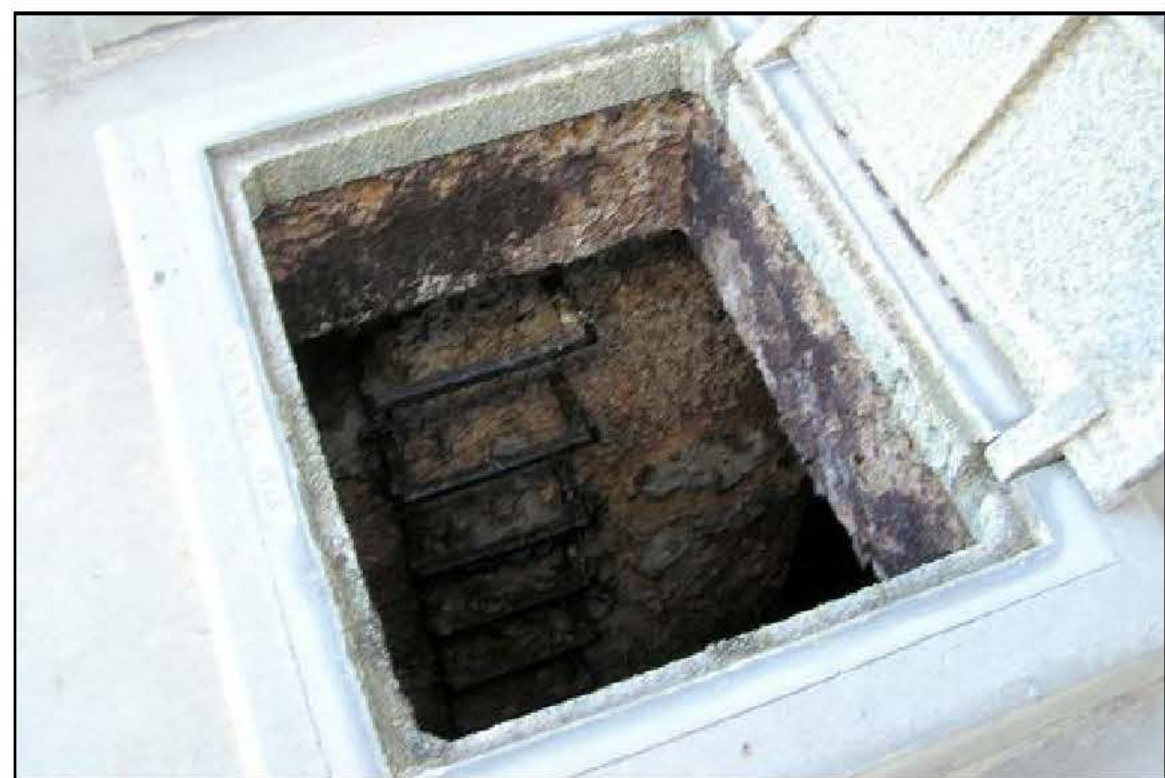
15 LOOKING EAST INSIDE WET WELL NO 1 AT EAST WALL AND ACCESS RUNGS
