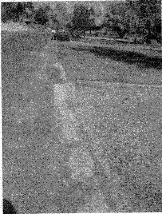
656 Young Street "gutter."
