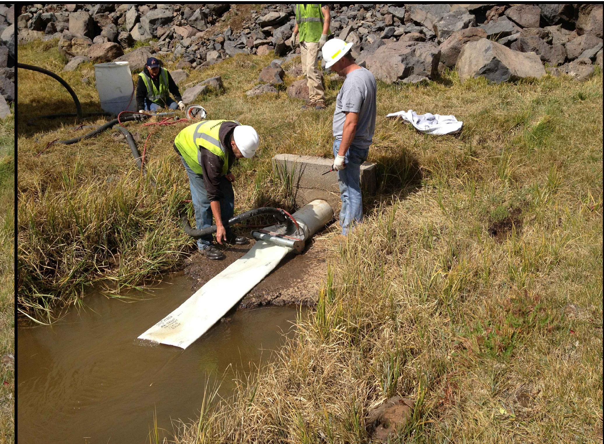
PHOTO 5: END OF INNER PORTION OF 2 PART LINER APPROACHING PIPE LINER AIR INVERSION TOOL AND PUSHED NEARLY ALL THE WAY BACK THROUGH THE OUTER LINER AND HOST PIPE TOWARD THE RESERVOIR SIDE. PHOTO AT THE OUTLET SIDE.
