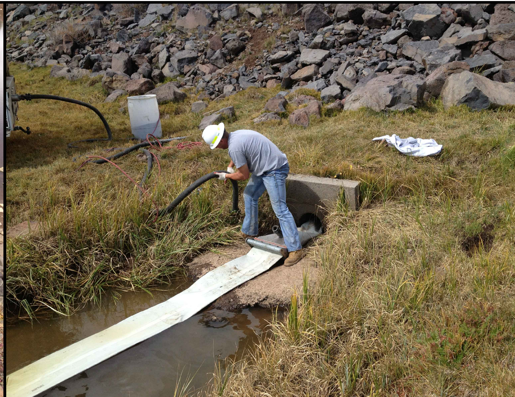
PHOTO 3: WORKER PREPPING INNER PORTION OF 2 PART LINER FROM OUTLET SIDE OF DAM TO BE PUSHED AND INVERTED BACK THROUGH THE OUTER PORTION PREVIOUSLY PULLED THROUGH THE HOST PIPE FROM THIS SIDE
