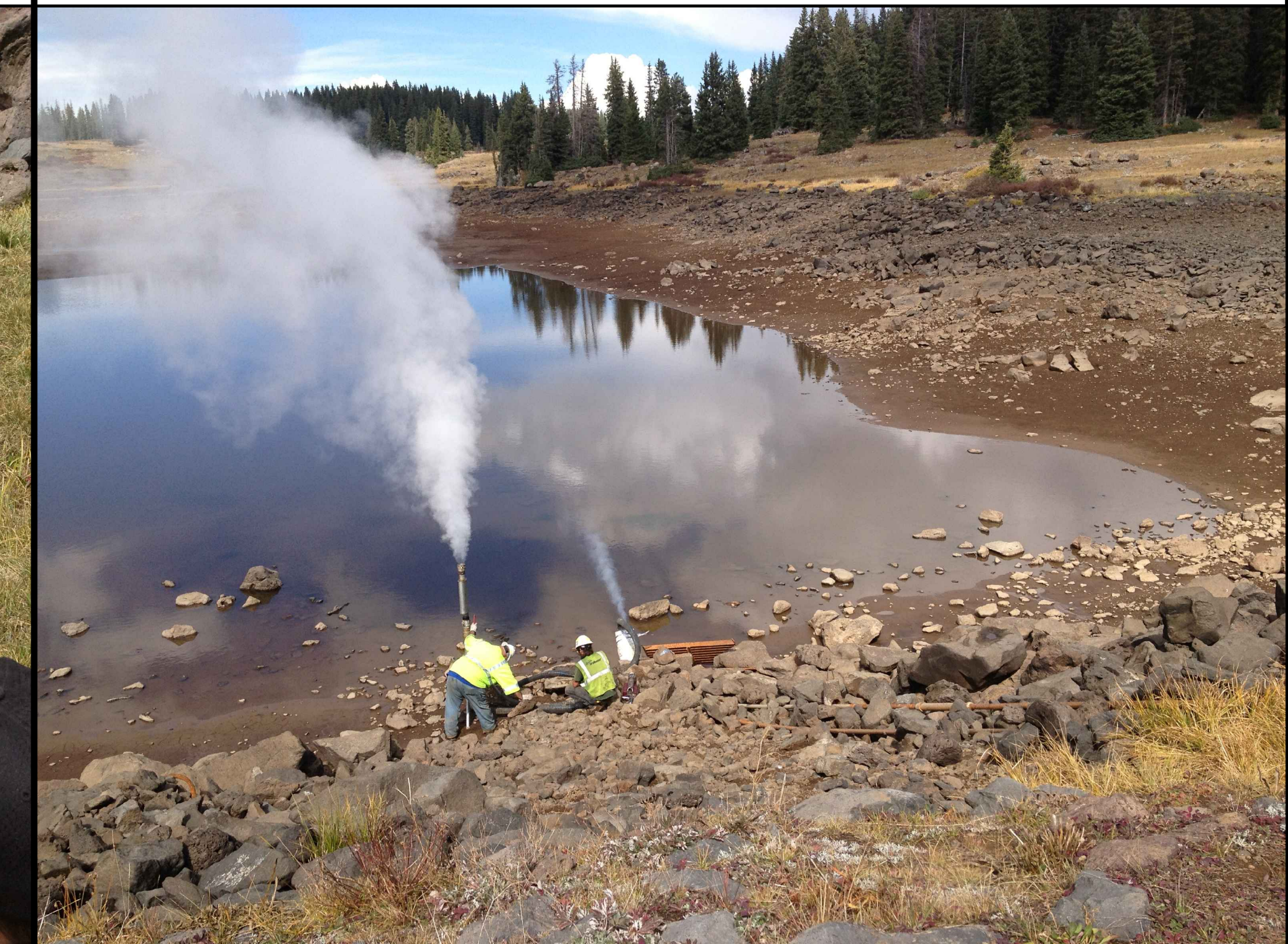
PHOTO 6: STEAM IS ADDED TO COMPRESSED AIR FROM A CONNECTION ON THE PIPE LINER AIR INVERSION TOOL (NOT SHOWN, BUT SHOWN IN PHOTO 5) TO ACTIVATE THE CATALYST CURING THE RESIN THEREBY COMPLETING THE CURED IN PIPE PROCESS FOR THE PROJECT
