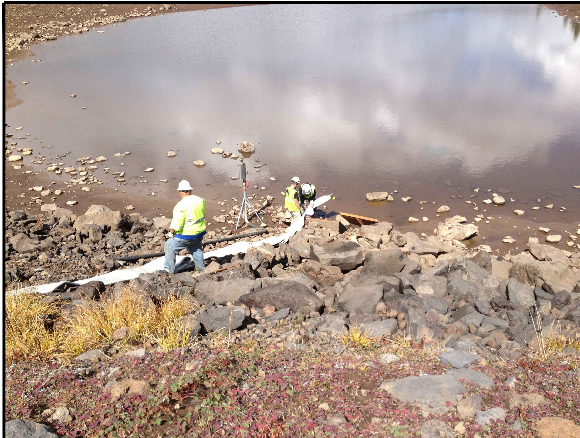
PHOTO 1: WORKERS PREPPING OUTER PORTION OF 2 PART LINER TO PULL THROUGH HOST PIPE FROM THE RESERVOIR OR INLET STRUCTURE END OF THE HOST PIPE.
