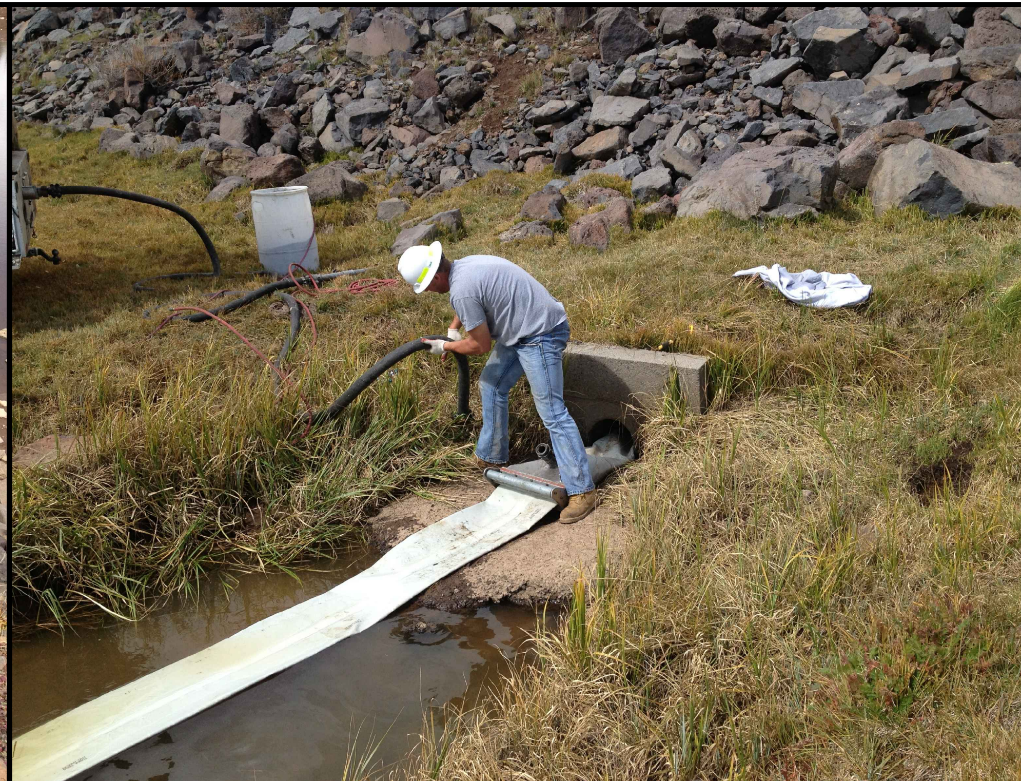
PHOTO 3: WORKER PREPPING INNER PORTION OF 2 PART LINER FROM OUTLET SIDE OF DAM TO BE PUSHED AND INVERTED BACK THROUGH THE OUTER PORTION WITH COMPRESSED AIR VIA A PIPE LINER AIR INVERSION TOOL. OUTER LINER PREVIOUSLY PULLED THROUGH THE HOST PIPE FROM THIS SIDE.
