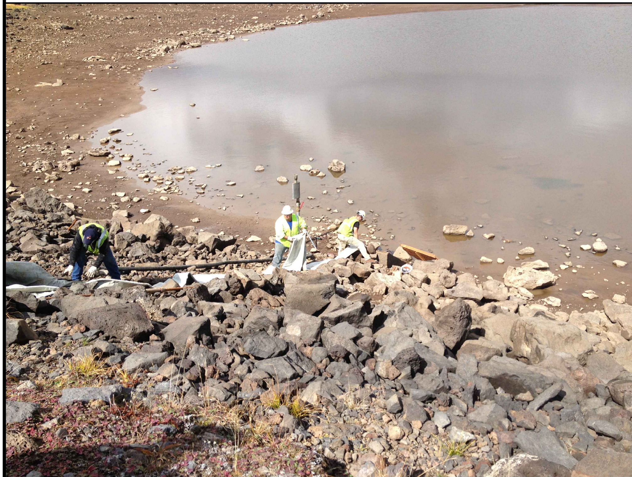
PHOTO 2: OUTER PORTION OF 2 PART LINER BEING FED THROUGH HOST PIPE FROM THE RESERVOIR OR INLET STRUCTURE END OF THE HOST PIPE AND PULLED FROM THE OUTLET END OF THE PIPE (NOT SHOWN).
